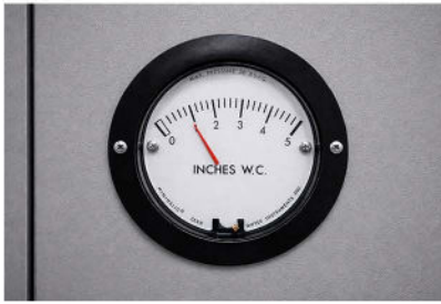
FIGURE 3 - DIRTY FILTER GAUGE
